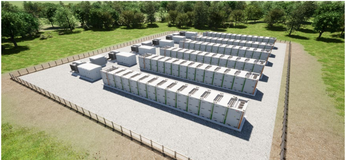
Image 4.7 Typical BESS Units
