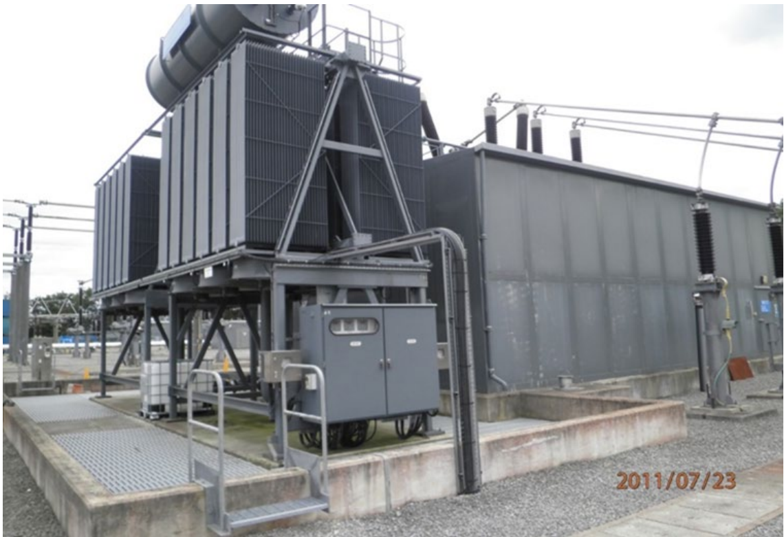
Image 4.5 Typical (large 400kV power transformer)
