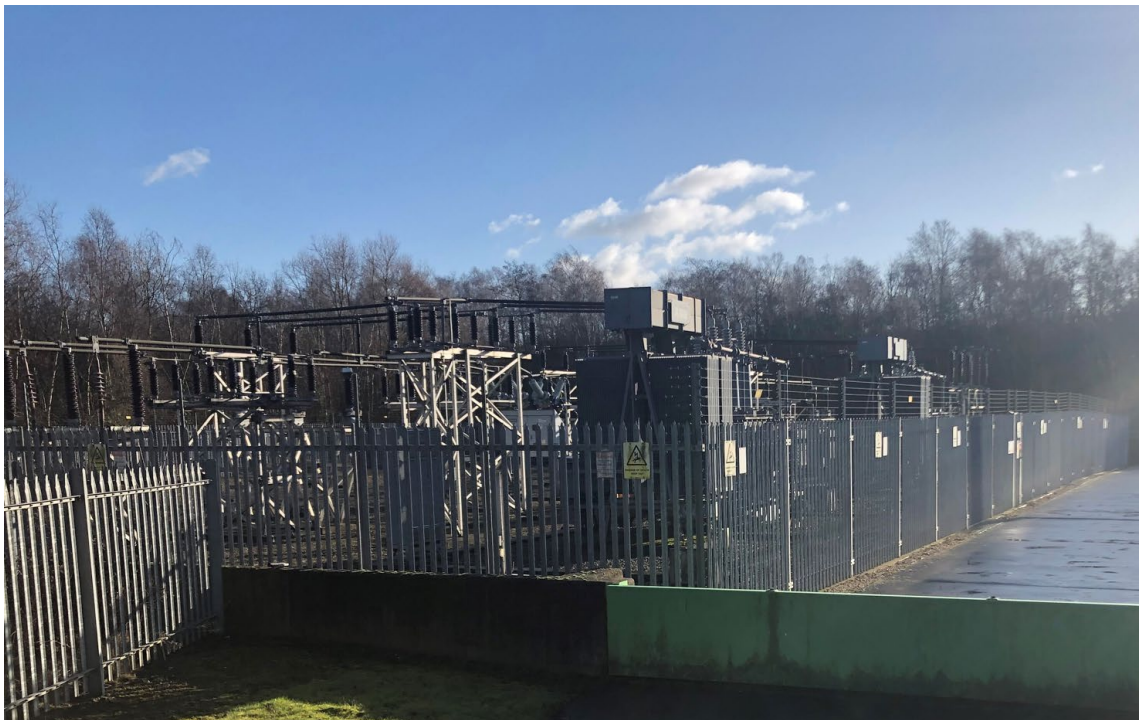
Image 4.6 Typical 132kV substation compound
